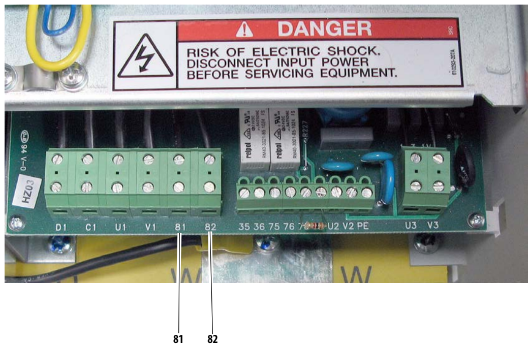
Figure 63 - Frame C Internal Armature Fuse Signal Terminal Block Location
