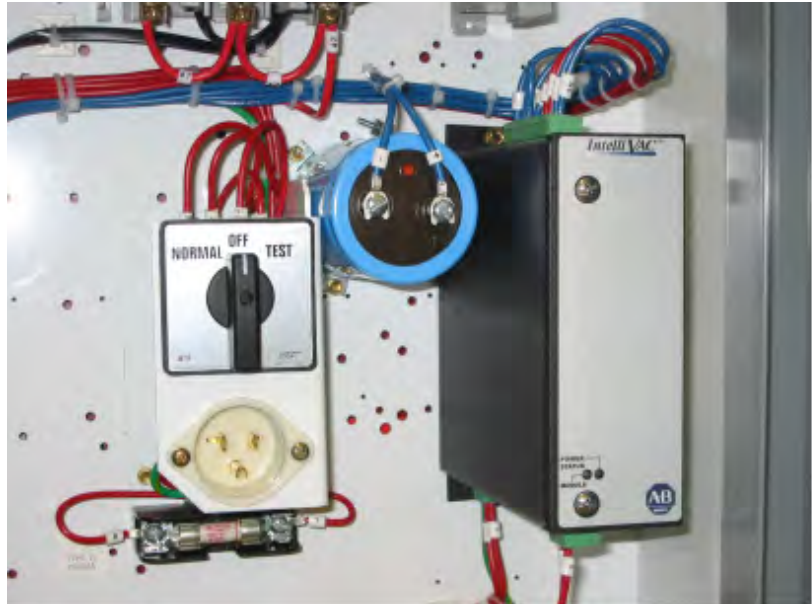
Figure 4 - Typical IntelliVAC Installation within a Bulletin 1500/1900 MV Controller (Shown with optional external capacitor)
